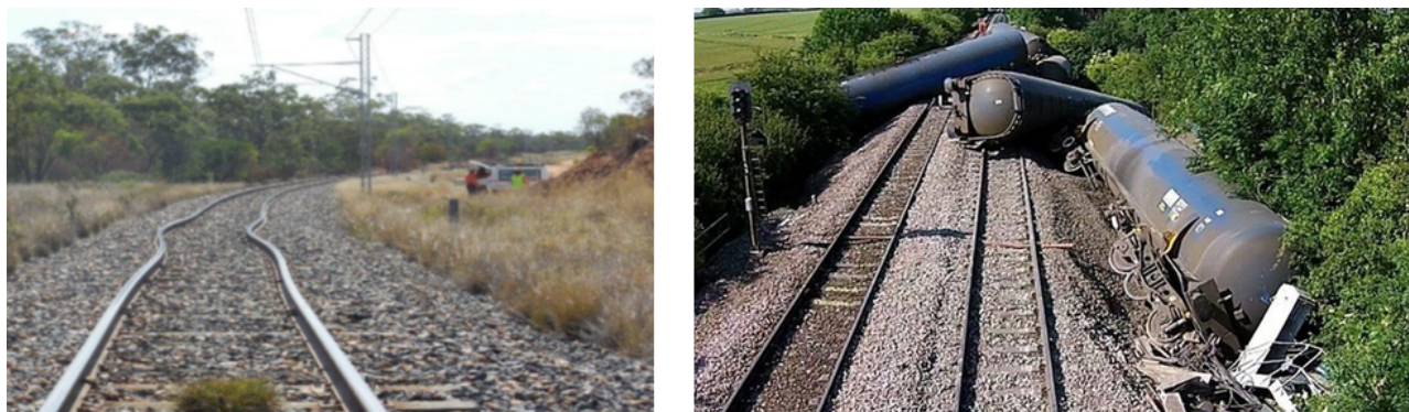
Figure 3-3: (left) Typical example of track buckle, Australia. (right) Train derailment due to heat induced buckling in Lincolnshire, UK
